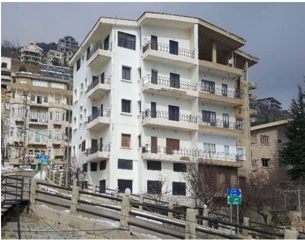
Figure 5.4 Picture showing building having the external envelope made of single CMU wall. Taken on: January 28th 2020 . Source: Author
