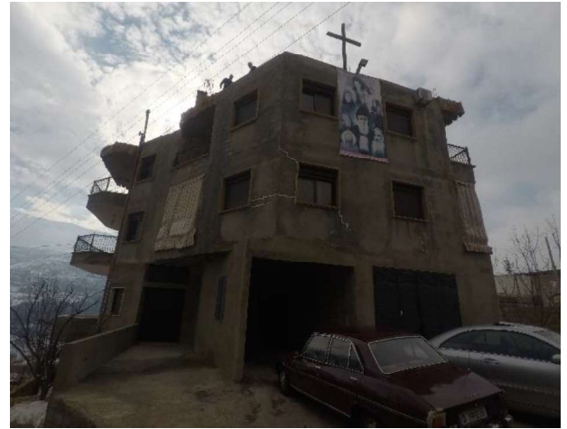
Figure 5.1 Picture showing building having the external envelope made of cavity wall. Taken on: January 28th 2020 . Source: Author
