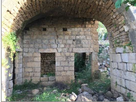
Figure 4.47 Leaks found in the house structure and the openings in the Liwan, Source: Author
