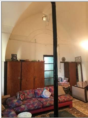
Figure 4.15 Photo of north- west room where the window is replaced by a door, Source: Author
