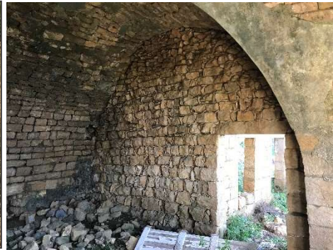
Figure 4.44 photo of the existing structure of the cross vault and the remaining plaster, Source: Author
