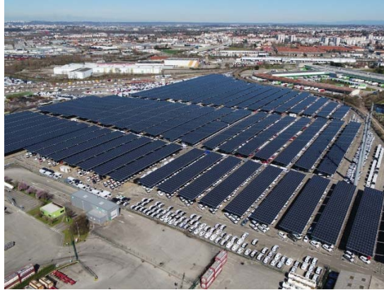
Figure 5.7 –Example of Solar Carports Installation: 16.3 MW solar array on a car park in Corbas, France The parking area around administration building will allow the installation of around 1900 photovoltaic modules as per Figure 5.8, 530W peak each, providing a total capacity of around 1MW peak.
