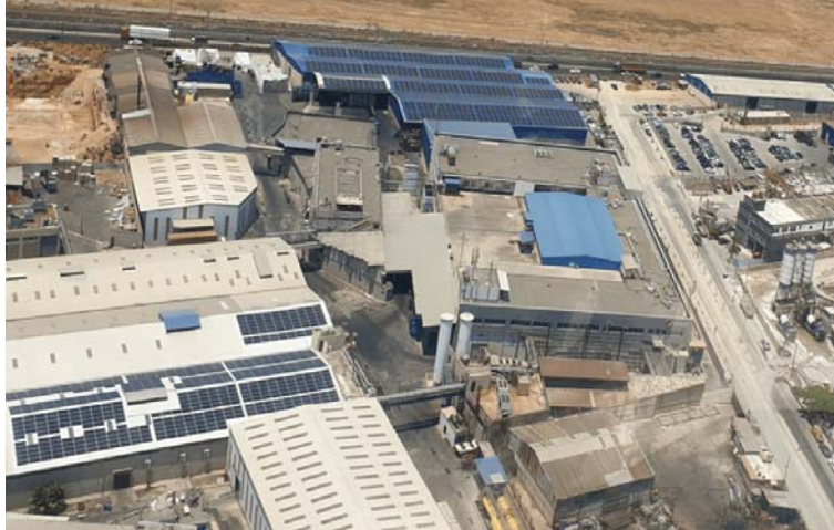
Figure 5.6 –Example of PV roof installation: SMLC PEPSICO Lebanon
