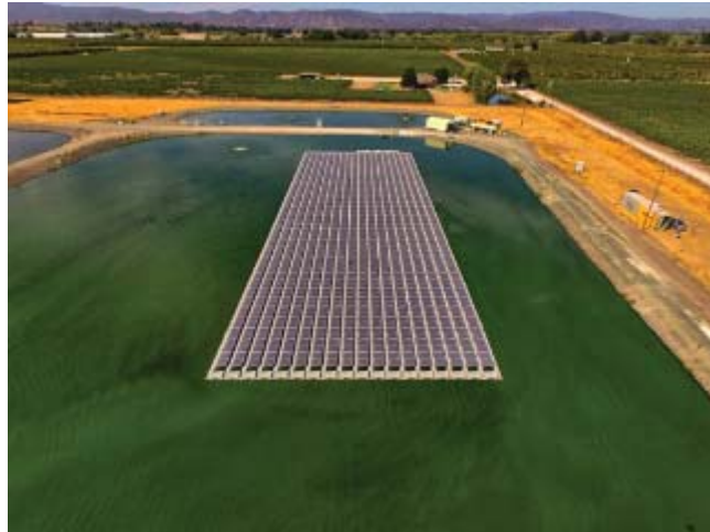
Figure 5.5 –Example of floating PV installation (Kelseyville country, California, USA, 252 kW)
